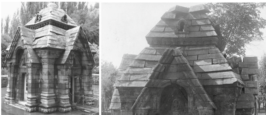
Fig. 7 The Pandrethan temple in 2006 (repaired in the twentieth century), with a close-up of the roof taken in 1903 after the 1885 earthquake. An earlier photograph in 1868 shows an identical misalignment of roof blocks ( Bilham et al. 2010 ) indicating that earthquakes before 1885 were responsible for the observed displacements
