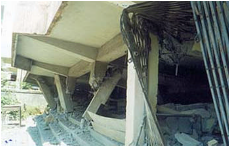
Photo 2: Shearing of load bearing base columns leading to the caving in of G+2 storied RCC structure, Naya Gaon, Port Blair
