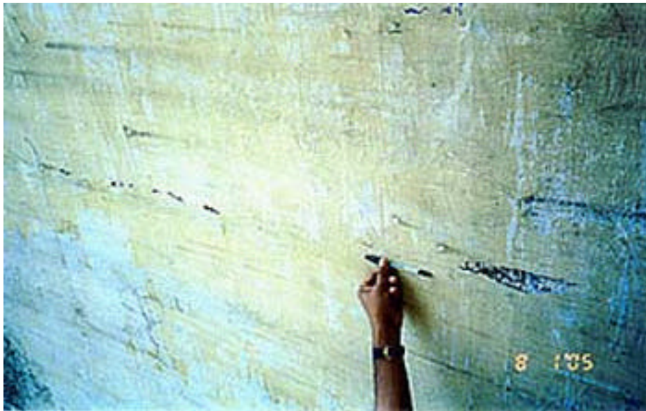
Photo 8: Fine cracks and chipping off plaster at the block joints of Dhanikhari concrete dam
