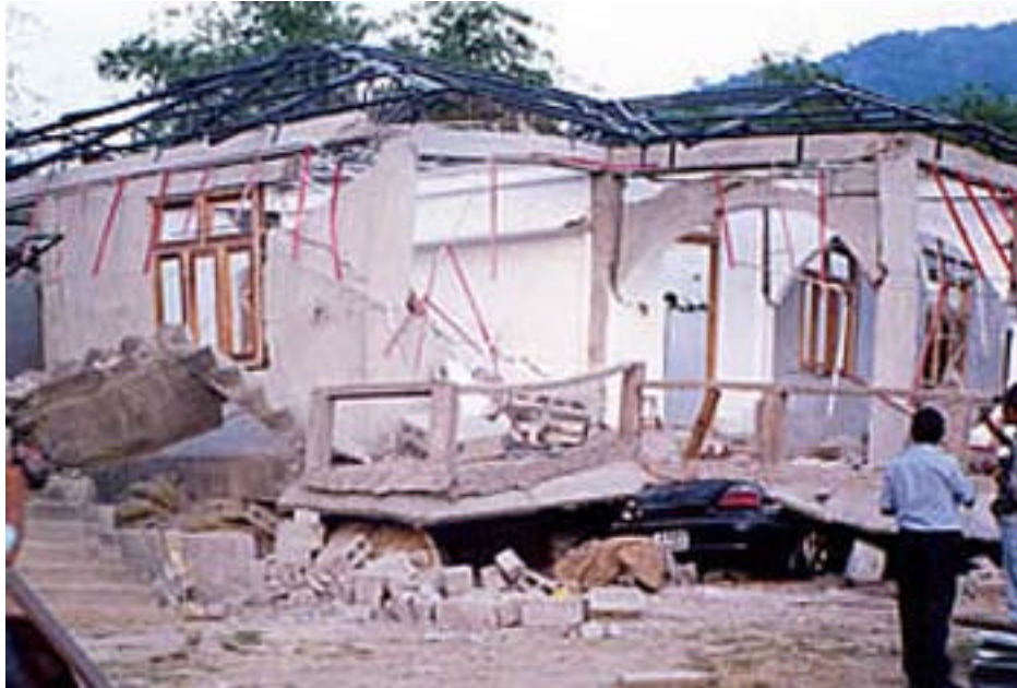
Photo 5: Complete caving in of the stilt and heavy damage of the first floor (now at ground floor level) of a newly constructed building in Kanyapuram. A car parked in the stilt got completely crushed
