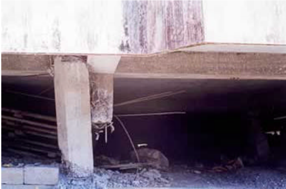
Photo 3: Sheared base column and caved in stilt, Naya Gaon,Port Blair
