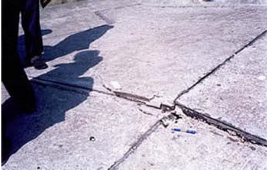
Photo 9: Buckling by 8 cm of the concrete apron at the interface of concrete spill way and earth section on the crest portion, Chouldari dam
