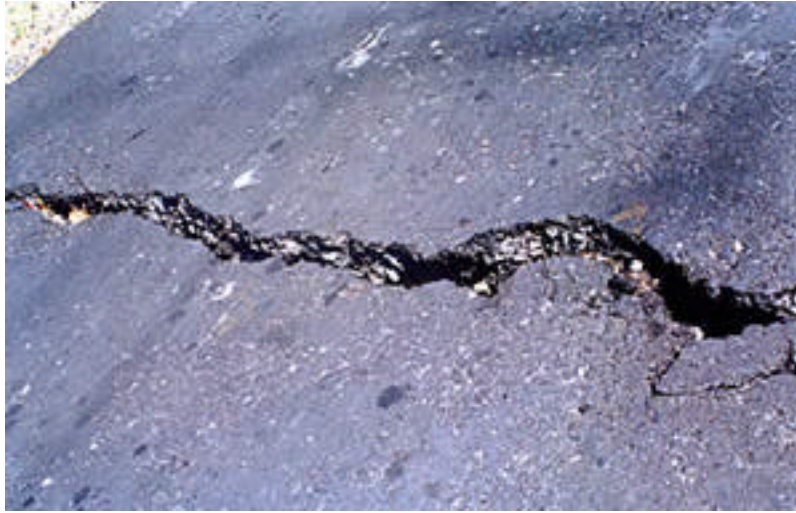
Photo 13: Fissure developed on the road at Baratang
