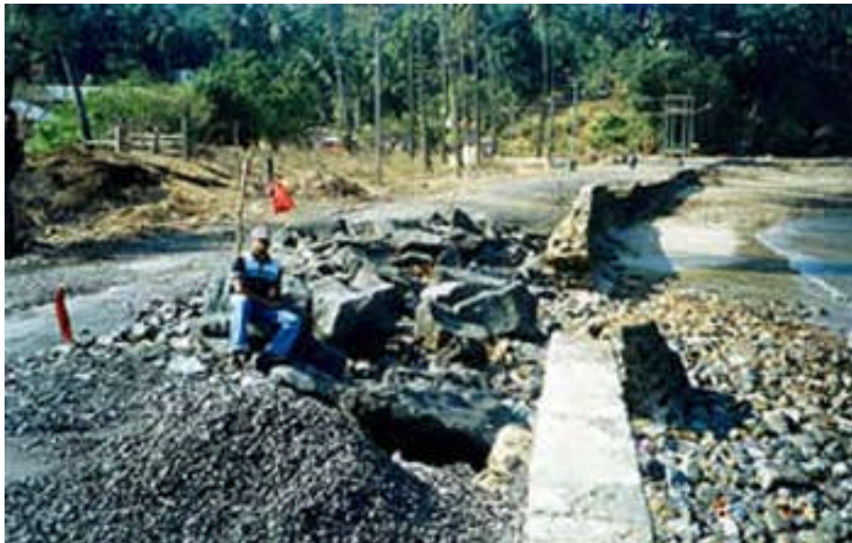
Photo 16: Breach in a section of the shore protection wall at Nazar, Port Blair
