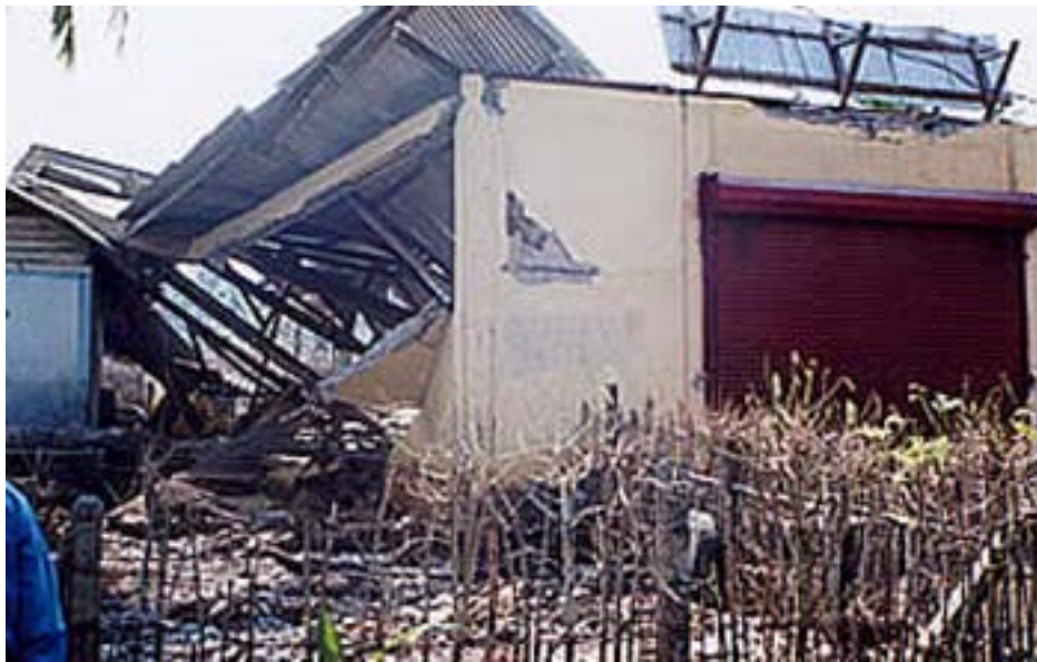
Photo 6: Failure of the three walls and roof of Malabar Society godown, Ograbraj due to strong tremors
