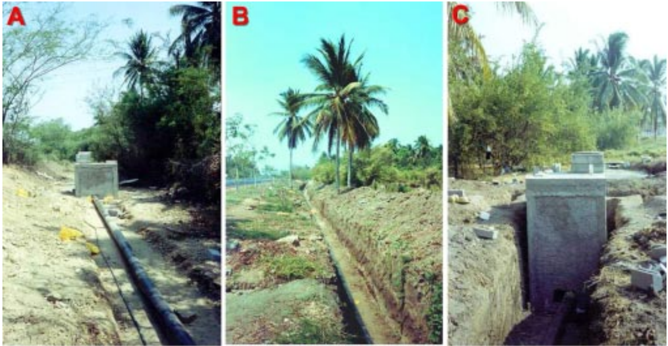
Fig. 9. Installation of the LBT. A – Polyethylene Ø8” pipe and the southern vault. B – Trench near the midpoint. The trench was accurately excavated and its bottom flattened using leveling control before pipe installation. C – Northern vault.
