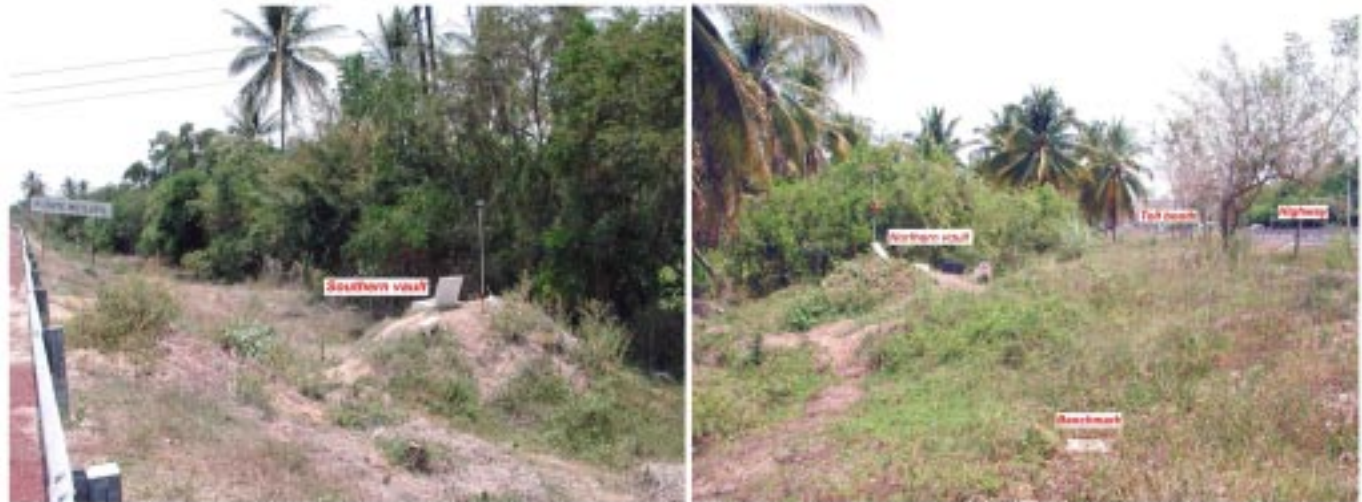
Fig. 10. LBT after installation. Left, southern vault. Right, northern vault with a benchmark in foreground and the highway tollbooth in the background. The vaults and the pipe are covered with at least 1 m topsoil to reduce temperature variation.
