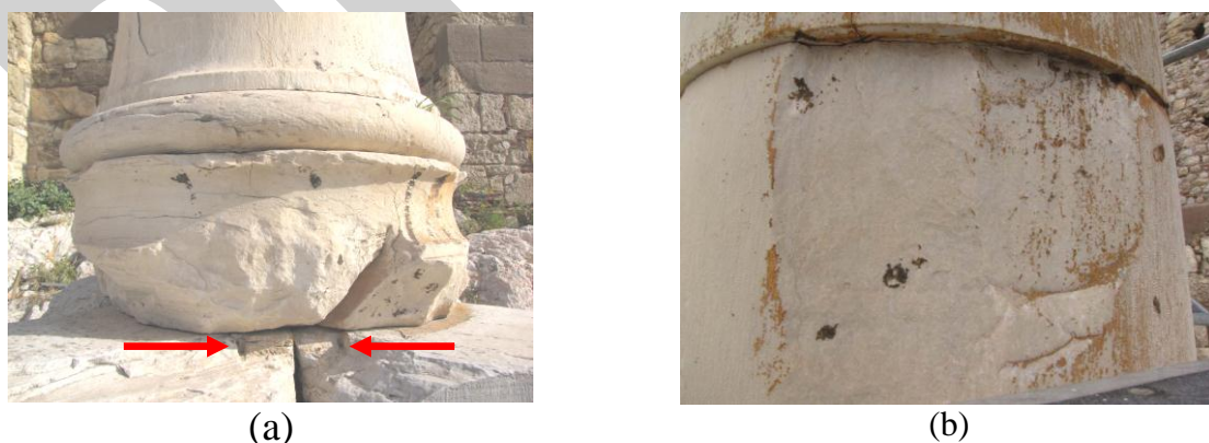
Figure 8. Column E: (a) Missing double-T clamp originally connecting the two pieces of the plinth (its position is shown between the two arrows); (b) Flaking off of skin of the stone of the 2 nd drum indicating rocking between 2 nd and 3 rd drums.
