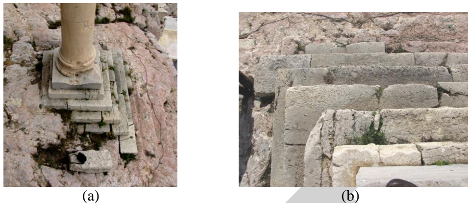
Figure 7. Column E: (a) Fragmented limestone stepped slabs of the pedestal; (b) View from above of the condition of the limestone stepped slabs of pedestal E (facing south).
