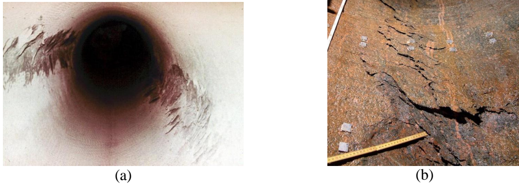
Figure 10. (a) Spalling of rock surface of tunnel wall with a tendency to shrink shortly after its formation; (b) Spalling of rock surface of bore hole (Courtesy Prof. D. Martin).
