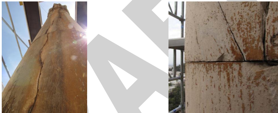
Figure 6. Typical damage to the shaft of column W caused by the oxidation and expansion of its dowels ( Zambas et al. 2011 ).
