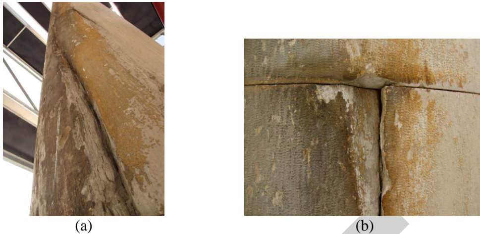
Figure 9. (a) Expansion of the stone and the formation of tension cracks due to oxidation of dowel(s) of the 5 th drum. Staining action caused by corrosive metals, Rust-colored bleeding can only occur from stone that contains a high concentration of iron pyrite; (b) Detail showing damage to the stone due to swelling of oxidized dowels enhanced by temperature effects. The expansion of the skin of the drum is arrested by frictional forces at its contact with the drum below.
